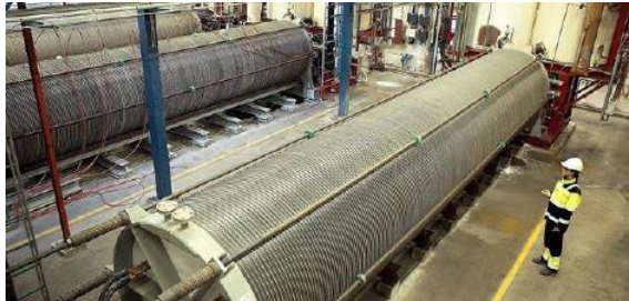
2.25 MW Alkaline Stack 43.3 kg/hr
